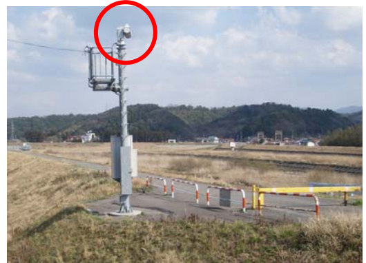
CCTV(河川巡視)
