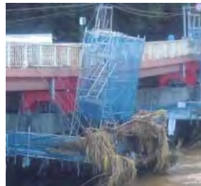
P2橋脚の沈下・傾斜
