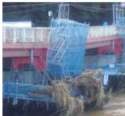
P2橋脚の沈下・傾斜
