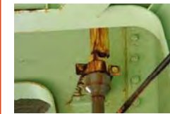
[排水管の欠損]
