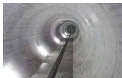
雨水貯留管(20,200m 3 )
