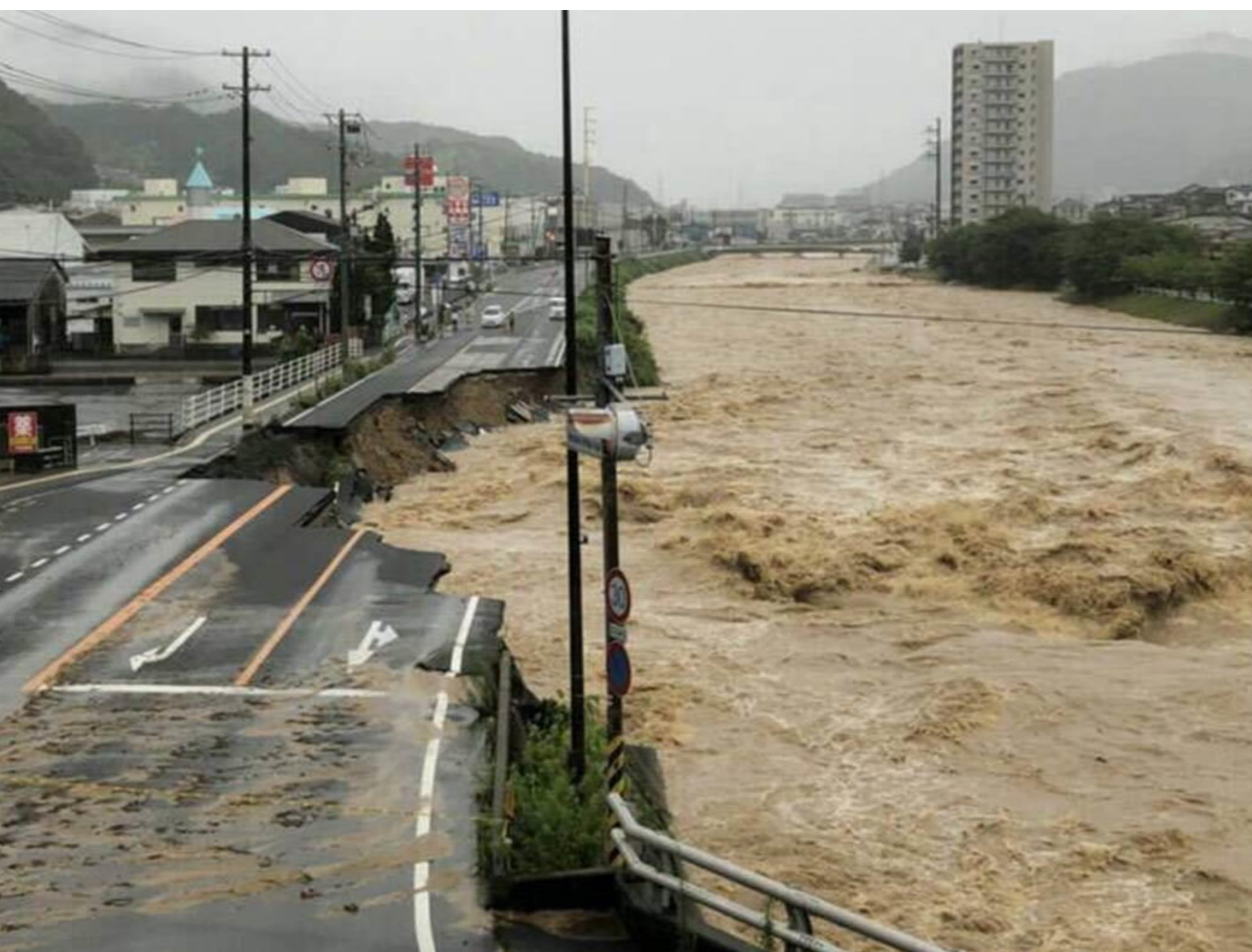
Traffic closed due to the loss of riverbank protection [Aki Ward, Hiroshima City, Hiroshima] (National Highway 2)
