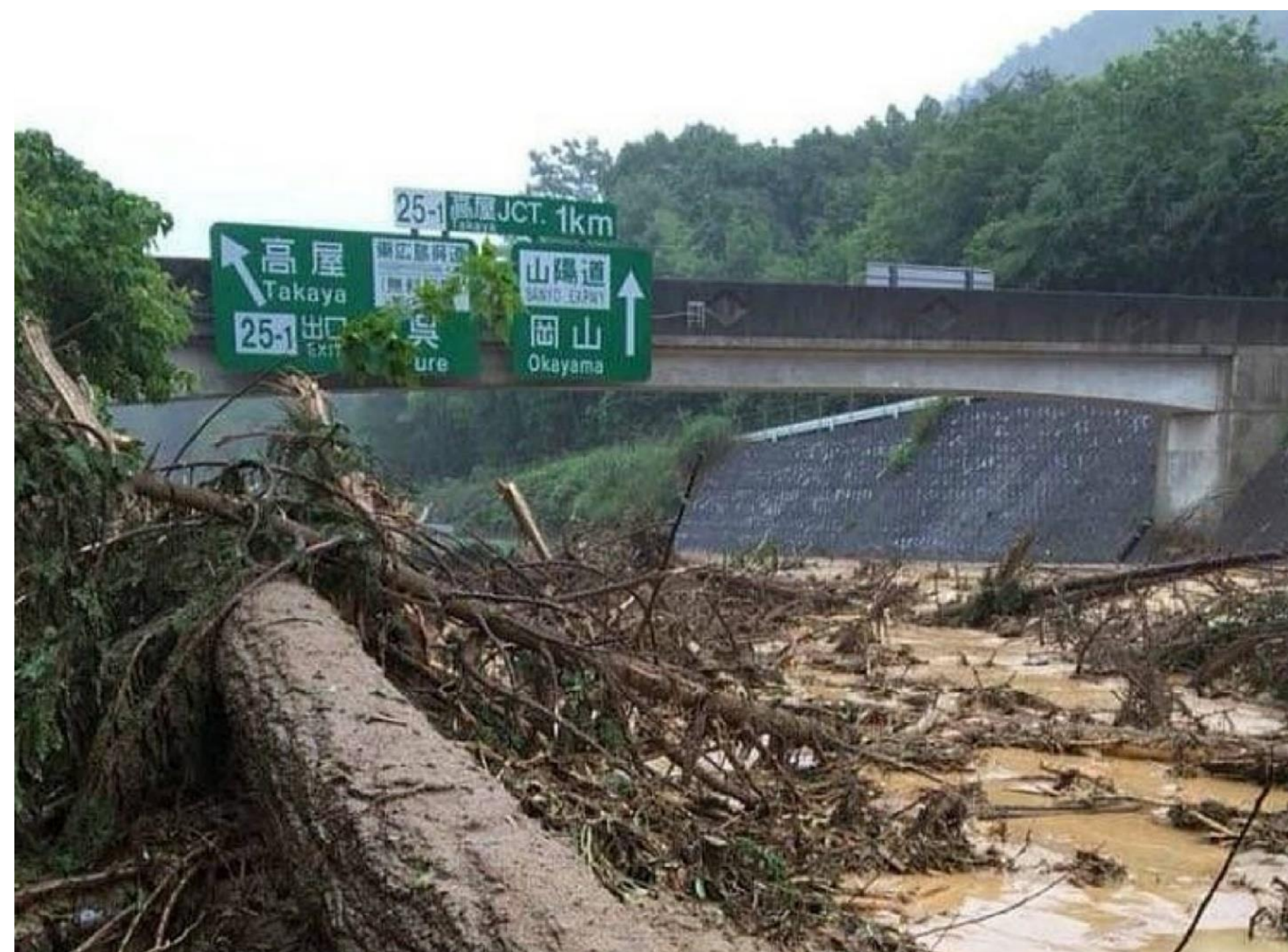
Mass washout and driftwood inflow out of the road [Higashihiroshima City, Hiroshima] (Sanyo Expressway (Around Takaya IC, JCT))
